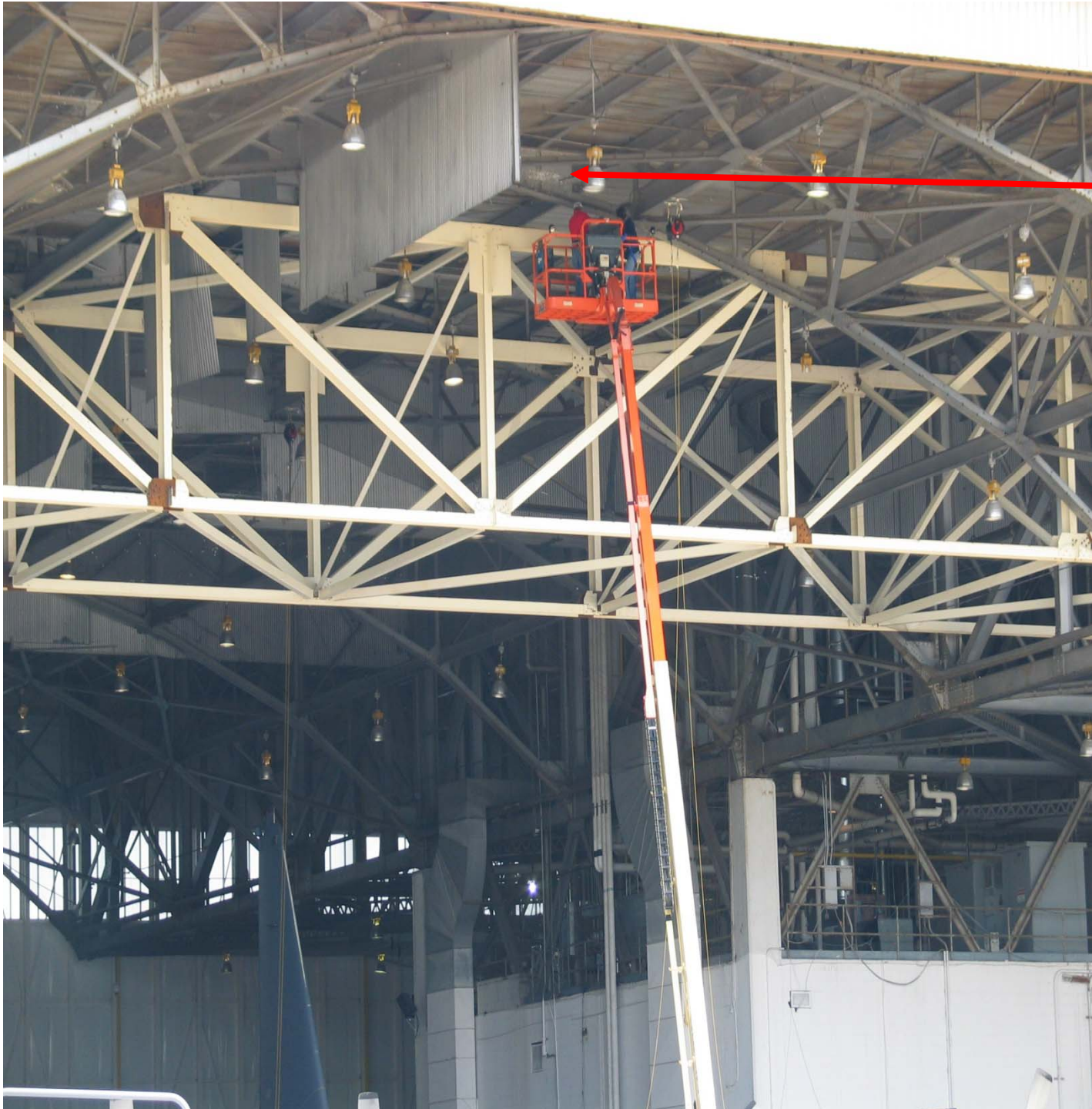
Bird remains being removed from Eason Hangar netting
